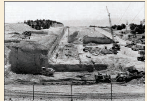
Excavation work for the Los Alamos Meson Physics Facility, on a finger-shaped mesa bordered by canyons to the north and south. (Image credit: Photo Los Alamos.)
